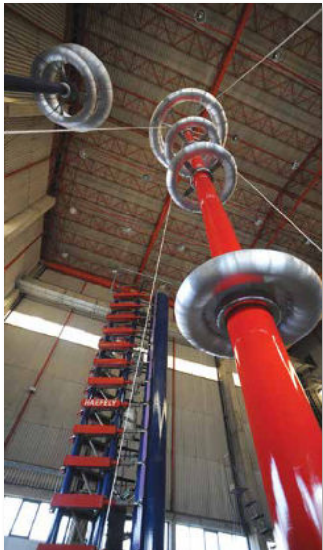
Lightning impulse generator voltage divider.
